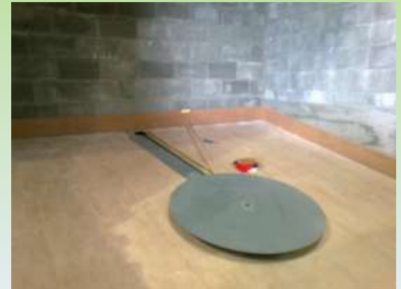
Pellet hopper and feed system
